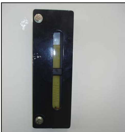
Hydraulic Tank Sight Glass
