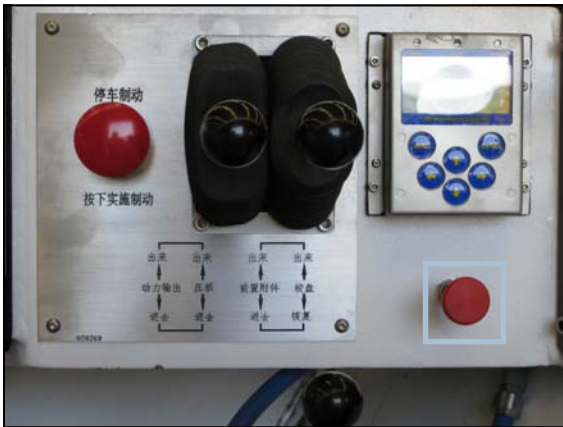
Emergency Intake Shut Off Valve Stop Button
