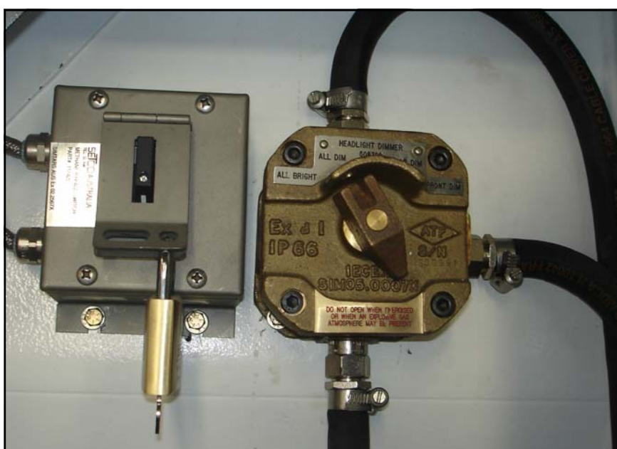
Manual Light Switch Box
